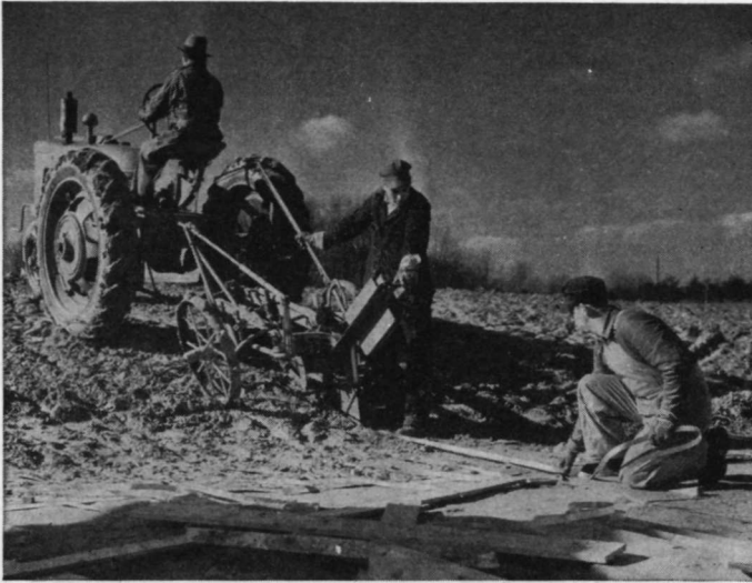
FIG. 2.67. A tractor-drawn wire plow for burying ground wires. The plow blade is of sheet steel that cuts a thin furrow. The wire is fed into the furrow as the plow advances. Horse-drawn hand plows of similar principle are often used.
