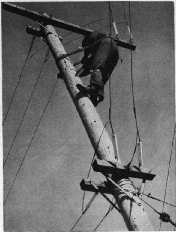
FIG. 4.83. Rigger working on a pole carrying balanced two-wire feeders for high-frequency broadcasting. This typifies many applications of this style of construction and hardware for broadcasting and communication use. This photograph was taken during construction, and the lines are not in final condition. Note the use of copper splicing sleeves at insulators, the attachment of guy wires, and crossarm hardware details. (Photograph courtesy of National Broadcasting Company.)
